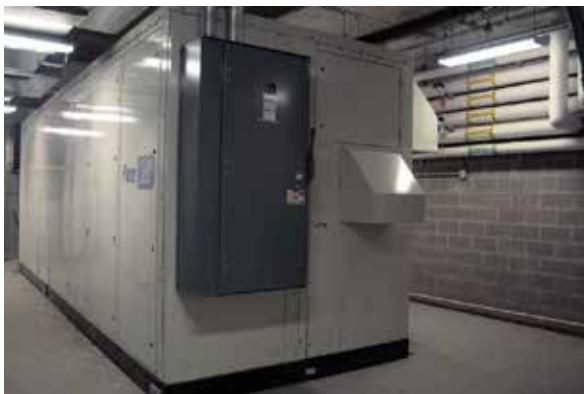
Apartment Investment Management Company's integration of Combined Heat and Power (CHP) technology in its 360 State Street apartment complex increased efficiency by 85 percent.
